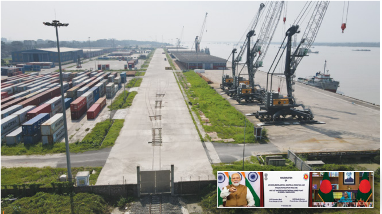
The Bank financed the construction of a 65 km broad gauge rail route, connecting Mongla Port to the existing rail network in Khulna, under the GOI-supported Line of Credit to the Government of Bangladesh, which was virtually inaugurated by the Prime Ministers of India and Bangladesh.
