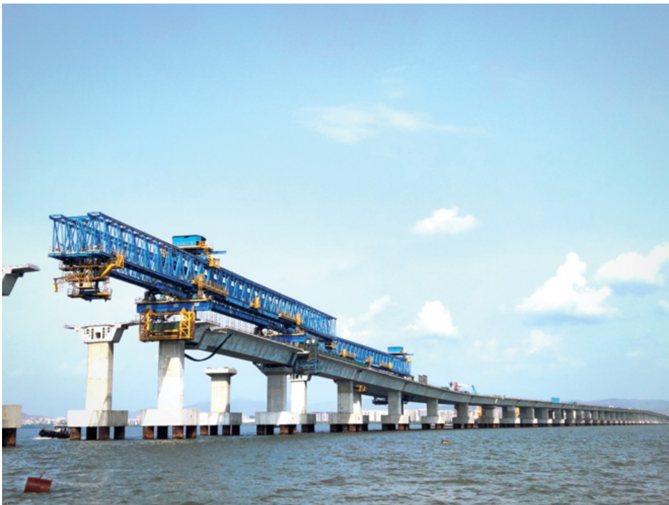
The Bank supported an Indian Engineering, Procurement and Construction (EPC) company for construction of a 7.8 km long bridge section, part of the Mumbai Trans Harbour Link.
