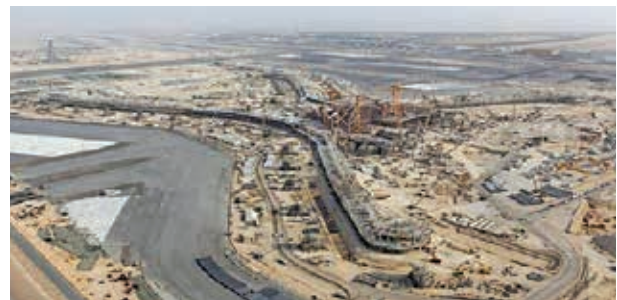
Exim Bank has supported Larsen & Toubro Ltd., for air side construction works for the new midfield terminal complex at the Abu Dhabi International Airport, UAE.
