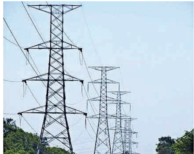
Construction of transmission lines connecting different regions in Lao PDR under a GOI Line of Credit of US$ 37.30 million.
