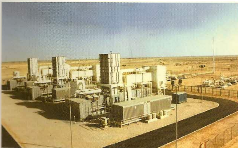
A view of Hubara Power Plant in Oman under execution by Bharat Heavy Electricals Ltd., New Delhi. Exim Bank has provided guarantees and bridge loans to the Indian company.
