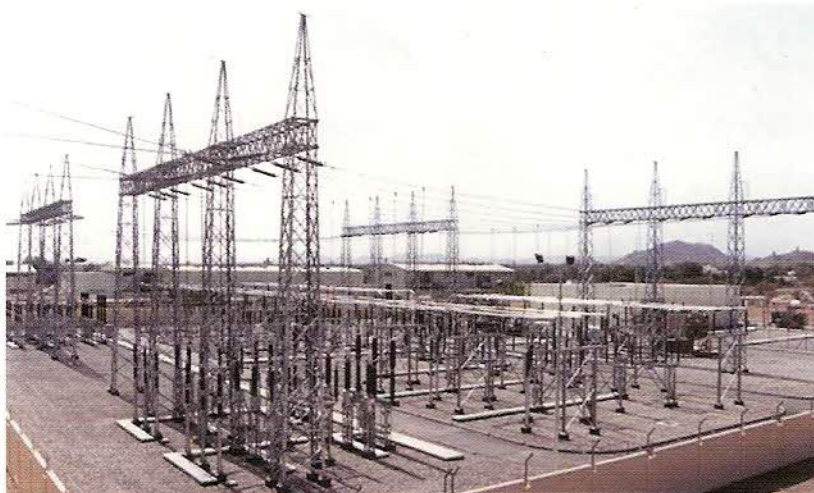
132 kV double circuit transmission lines and substation in Sharqiya Region, Oman, executed by Jyoti Structures Ltd., Mumbai. Exim Bank has provided guarantees and bridge loans to the Indian company.
