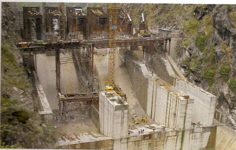
92 metre high Concrete Gravity Dam under construction at Tala Hydro-Electric project, in Bhutan, being executed by four Indian project export companies viz. Larsen & Toubro Ltd., Jaiprakash Industries Ltd., Hindustan Construction Company Ltd. and Bharat Heavy Electricals Ltd.
