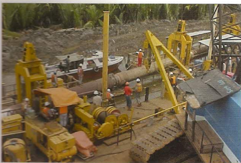
Gas Pipeline Project under construction in Indonesia by Punj Lloyd Ltd., New Delhi. Exim Bank has provided guarantees and bridge loans to the Indian company.
