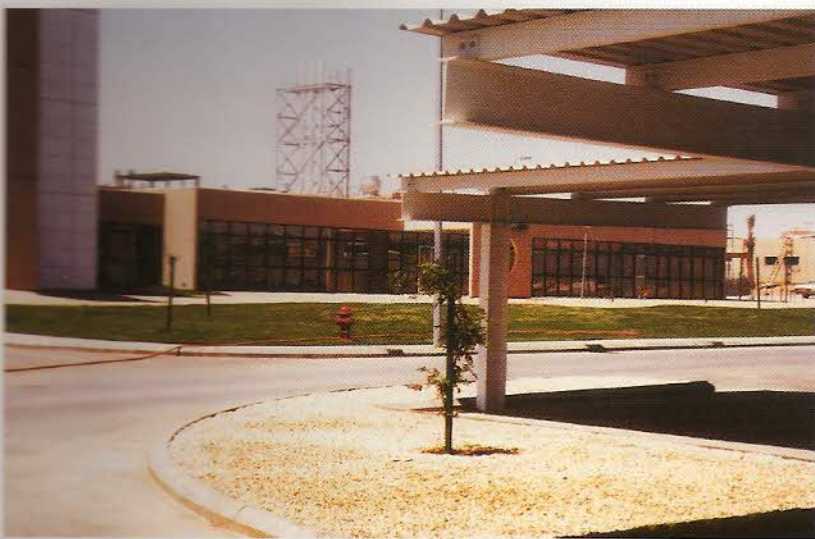
One of the three 100 bed super-speciality hospitals under construction in Saudi Arabia by Larsen & Toubro Ltd., Chennai and Progressive Constructions Ltd., Hyderabad. Exim Bank has extended guarantee support to the Indian companies.
