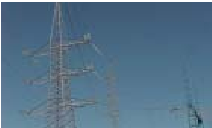
KEC International Ltd. (KEC) is one of the largest power transmission turnkey contractors in the world, having constructed over 35,000 km of transmission lines, worldwide. Seen above is the 90/150/225/400 KV 660 km transmission line in Tunisia for Société Tunisienne de l'Electricité et Gaz. Exim Bank has provided guarantees and loans to KEC.
