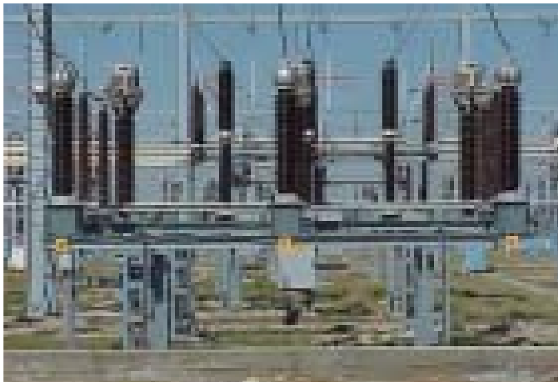
Bharat Heavy Electricals Ltd. (BHEL) which ranks among the major power plant equipment suppliers in the world, is one of the largest turnkey exporters of engineering products and services from India in the energy infrastructure sector. A view of 4x156.1 MW Al-Jabal Al-Gharbi Gas Turbine based Power Project (West Mountain Gas Power Project) in Libya under execution by BHEL for General Electric Company of Libya. Exim Bank has provided guarantees and loans to the company.
