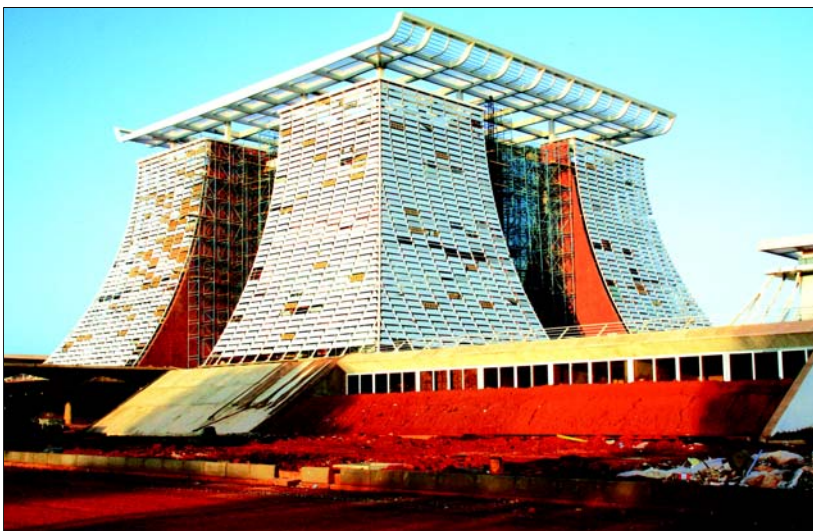
President's office and the seat of the Government under construction in Accra, Ghana, by the Indian project contractor M/s Shapoorji Pallonji & Co. under a US$ 60 mn Line of Credit from Exim Bank to Govt. of Ghana.
