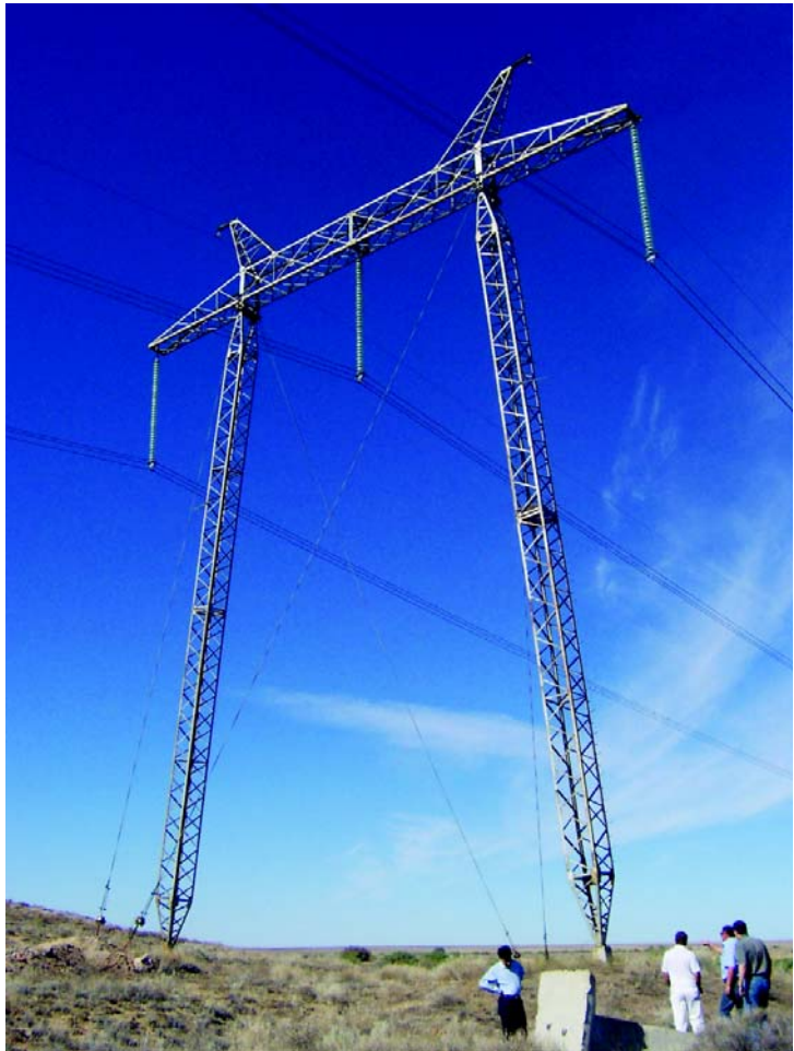
Turnkey project for supply and erection of 500 kv Single Circuit suspension tower in Kazakhstan executed by KEC International Ltd., Mumbai, assisted under Exim Bank's programme for project exports.
