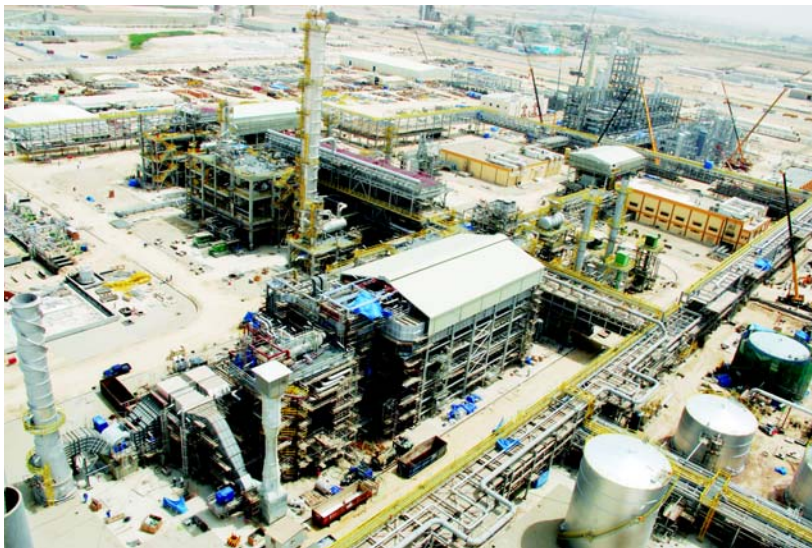
Turnkey project for methanol and carbon monoxide plant at Al-Jubail for Saudi Formaldehyde Chemical Co. Ltd., being executed by Larsen & Toubro Ltd., Mumbai, with financial support from Exim Bank.
