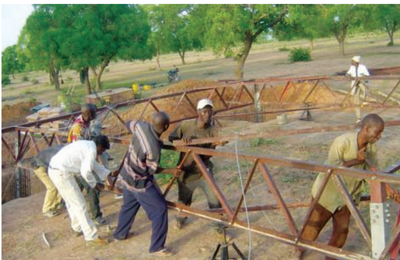
Construction of 225 KV Interconnection High Voltage Transmission Line between Mali and Cote d'Ivoire, being executed under Government of India supported Exim Bank's Line of Credit of US$ 45 mn to Government of Mali.
