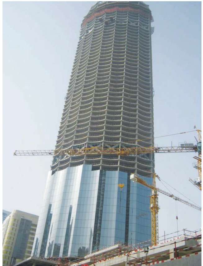
Turnkey contract for installation, servicing and maintenance of T2 and T3 tower under Central Market Redevelopment Project, Abu Dhabi, being executed by Voltas Limited, Mumbai, assisted under Exim Bank's programme for project exports.
